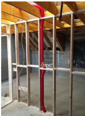
Radial pipe going through timber stud wall (recommended to use a minimum of 100mm wide timber).
