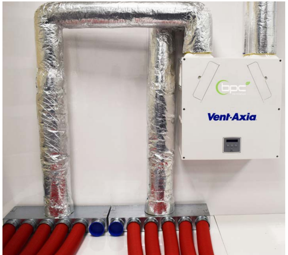
Unit and distribution boxes completed.
